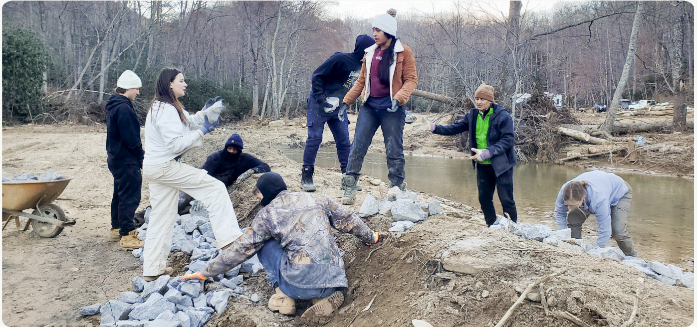
The team of volunteers moves boulders and debris from a flood-affected yard in North Carolina
